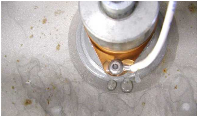
Illustration 15.2. Leaking tank floor with traces of liquid
